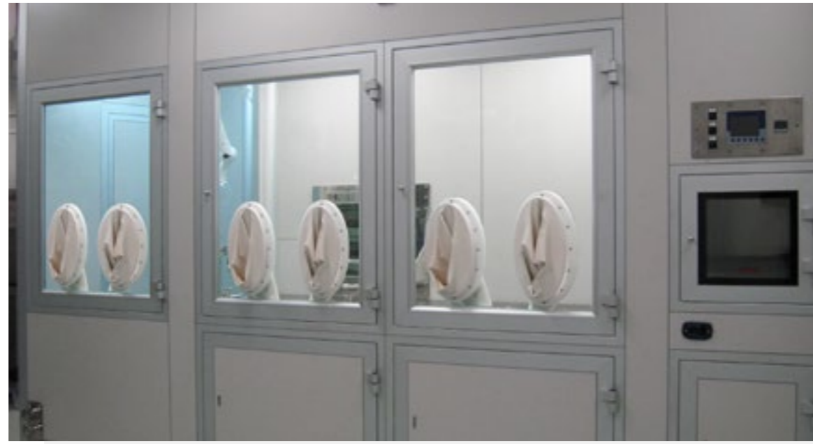
RABS (Restricted Access Barrier System) con pareti Nicomac e pass-box
